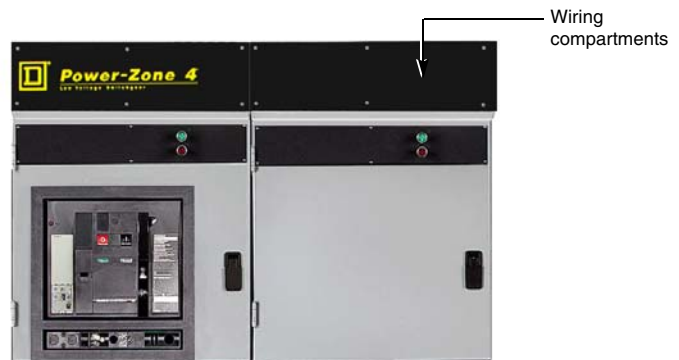
Figure 34: Removing the Wiring Compartment Covers
